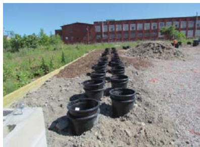
From Left: Orange visual barrier, 3/4" crushed stone drainage layer, 6-8" barrow material and insert/socket pot growing system.
